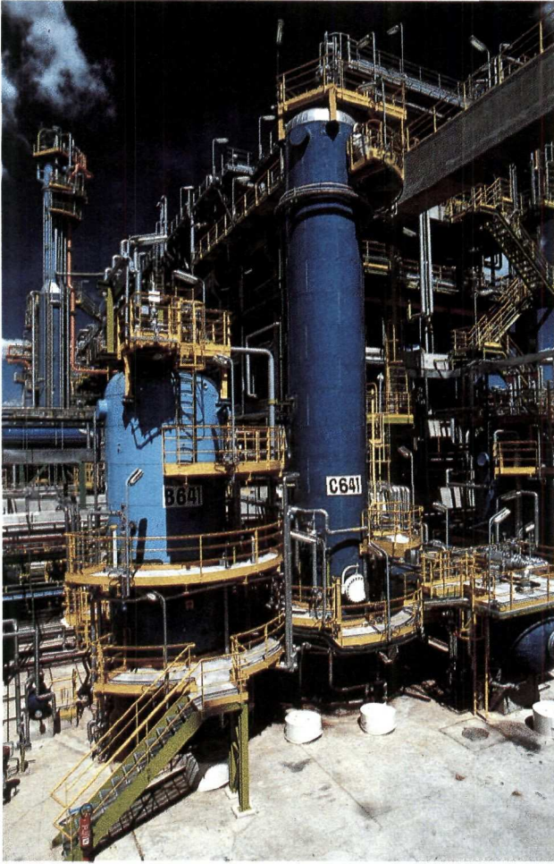
Raffinerie de Provence - Gas Plant
